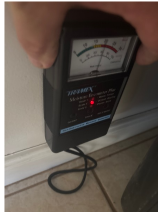
Moisture behind main shower
