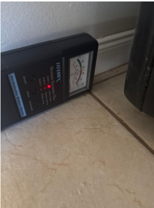
Moisture behind main shower
