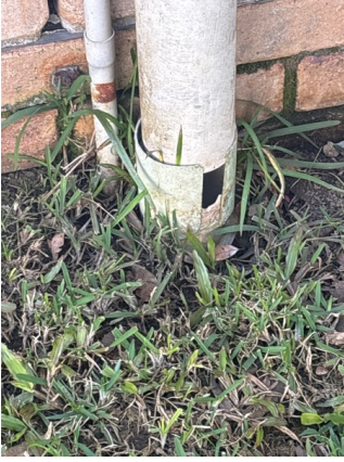
Broken down pipe
