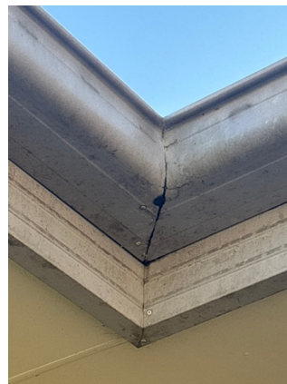
Leaking gutter join
